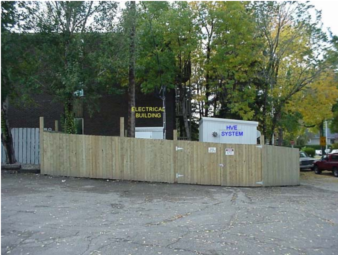
FIGURE 5. The major surface facilities for the ET-DSP and high vacuum dual phase extraction system were located next to the apartment building. The area was fenced off for safety and operational reasons. Power lines, hoses, and extraction piping were all placed below ground to ensure that the esthetic value of the site was maintained during remediation operations.
