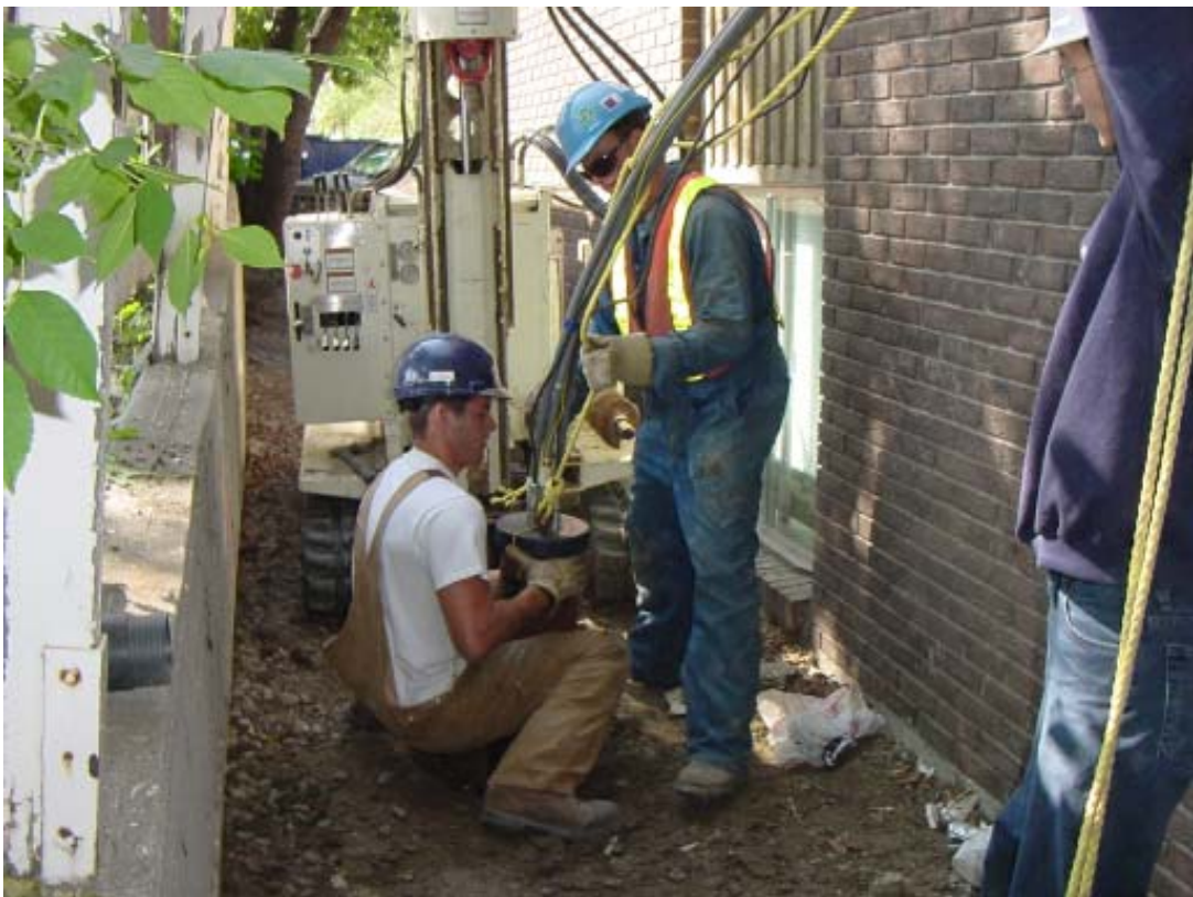
FIGURE 7. Specialized drilling methods were used to drill well locations in limited access areas.
